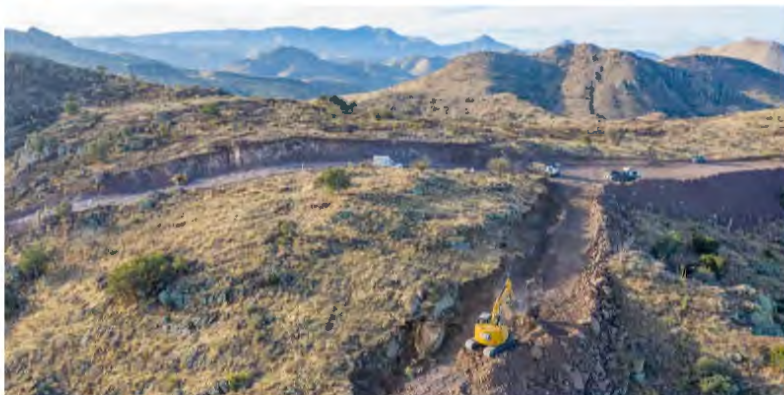
Construction machinery at a standstill, in Guadalupe Canyon at the Arizona-New Mexico border, on January 20 2021. John Darwin Kurc
